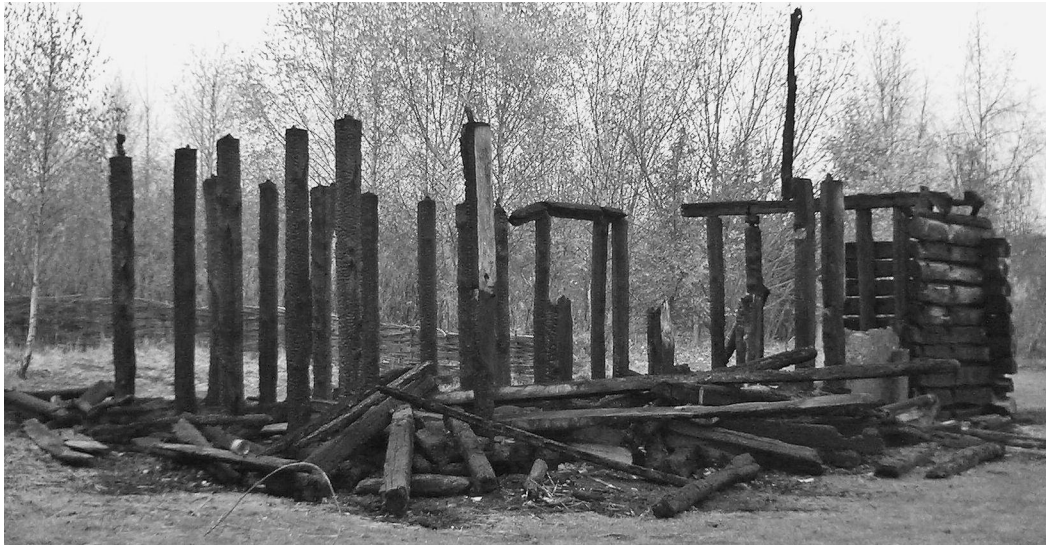
Fig. 2 Remains of the hall building after the 2008 fire; viewed from the south-east corner (photograph by Christine Elgy)
